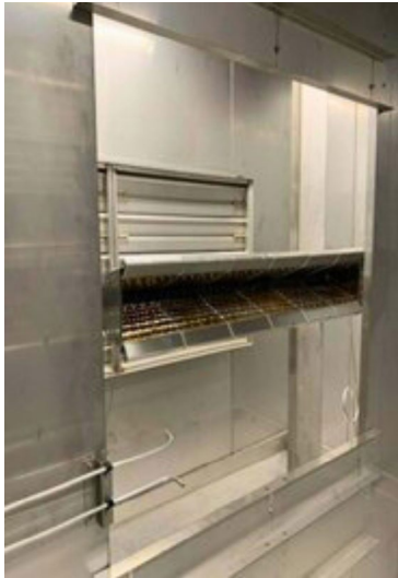
Direct Fired Burner
