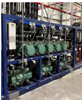
Refrigeration Control System Integration
