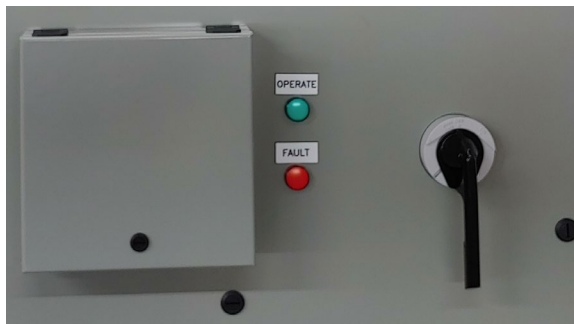
Main Disconnect in OFF Position
