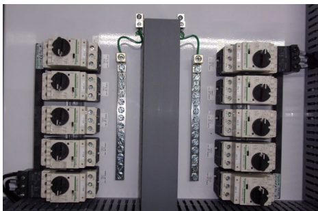
MMP in Control Panel
