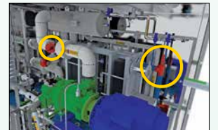
Compressor Isolation Valves
