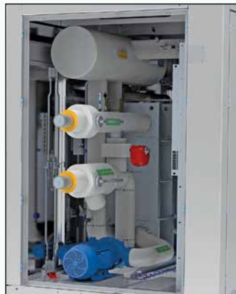
Chilled fluid pump, valves & bypass for chilled loop
