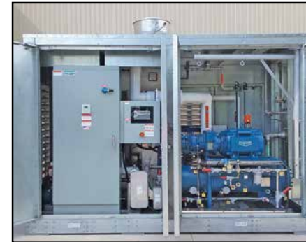
Front view showing compressor package, unit power panel and HMI
