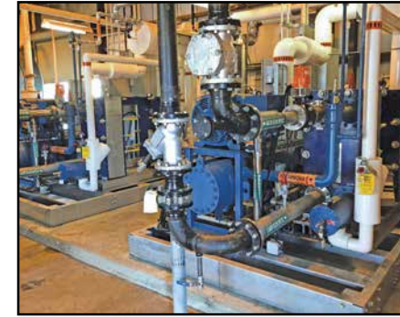
Indoor chemical plant application without enclosure
