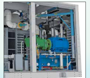
Rigging Davit for Compressor and Motor Removal
