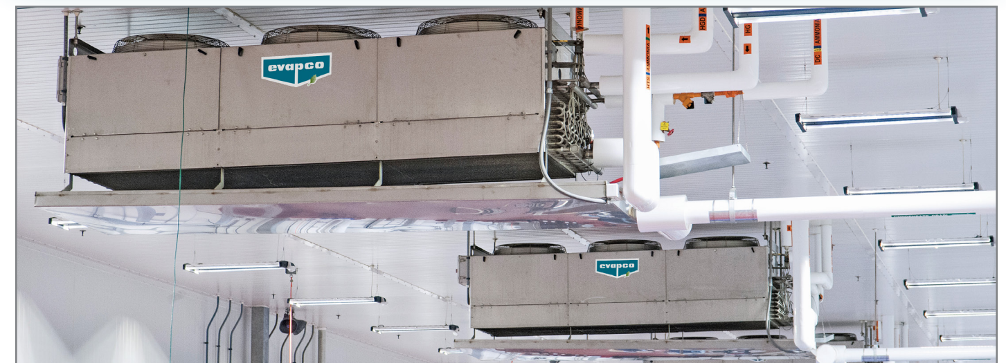
SSTWE Work-Room Evaporators
