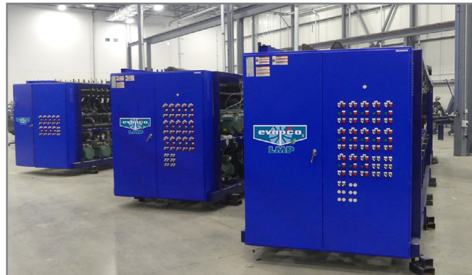
Purity Rack Highlighting Microprocessor Control Panels
