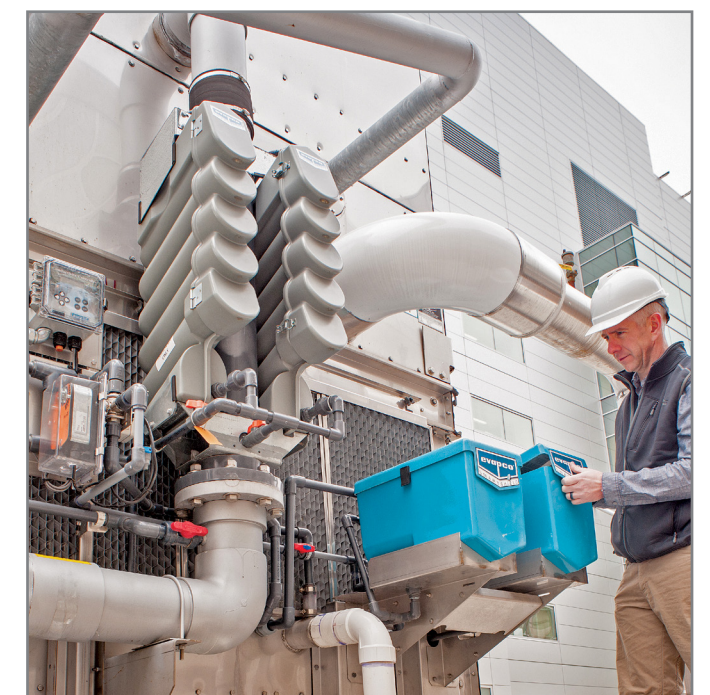
Smart Shield® Factory-Mounted Water Treatment System
