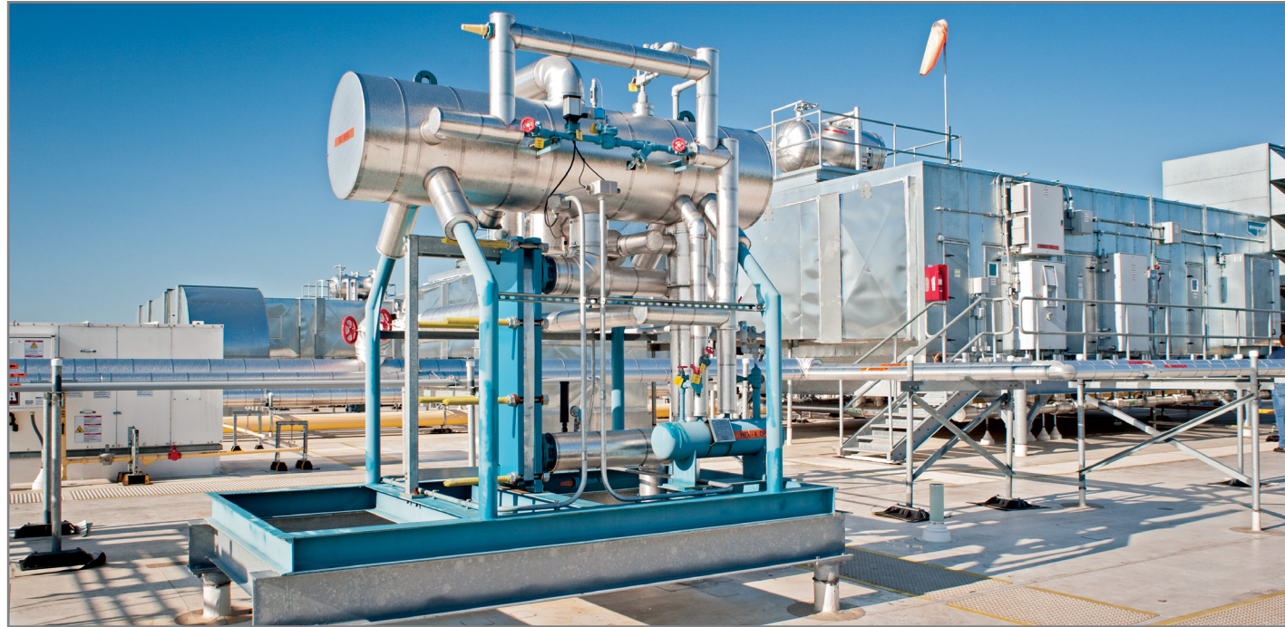
RVS MPC Chiller Package
