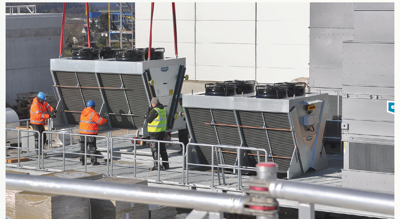
EVAPCO Air Solutions V Series, Germany
