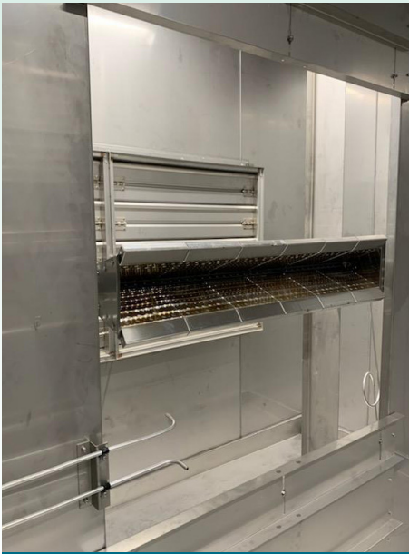
Direct Fired Burner
