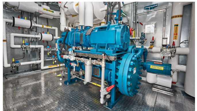
Low Charge Ammonia Machinery Room LCR-P-W
