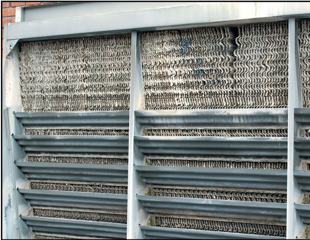
Old, Inefficient, Damaged Fill
