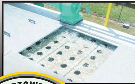
Hot Water Basins
