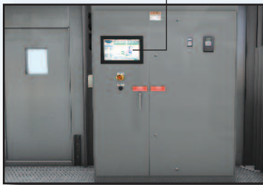
Main Control Panel – Interior View
