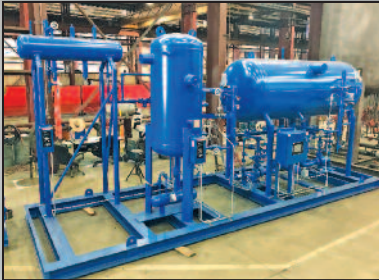
Refrigeration Skid Package
