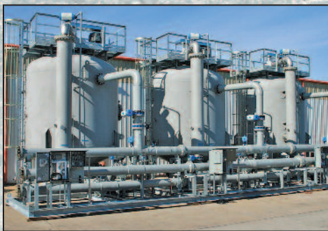
Water Filtration Skid
